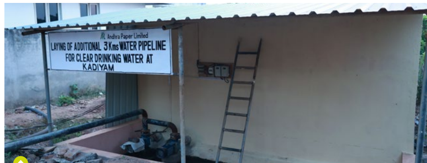
Laid 3 Kms. pipeline providing drinking water facility to the villagers of Kadiyam, East Godavari District
