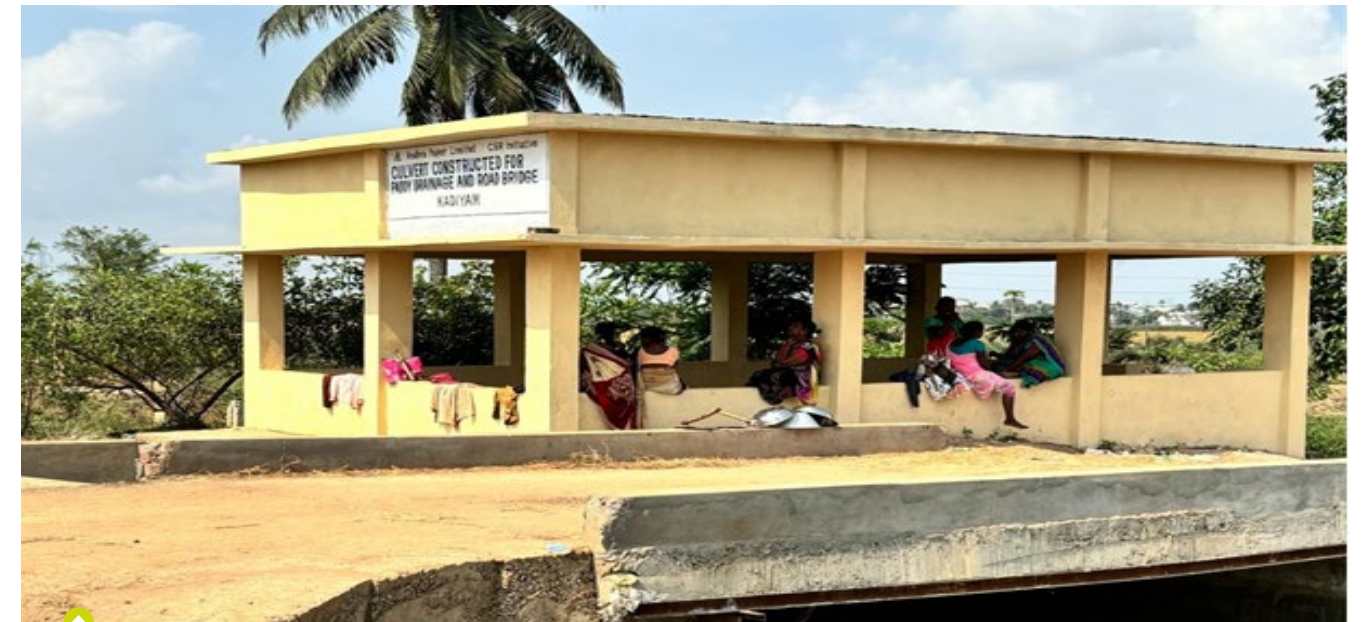
Culvert construction for paddy drainage and road bridge, Kadiyam Mandal, East Godavari
